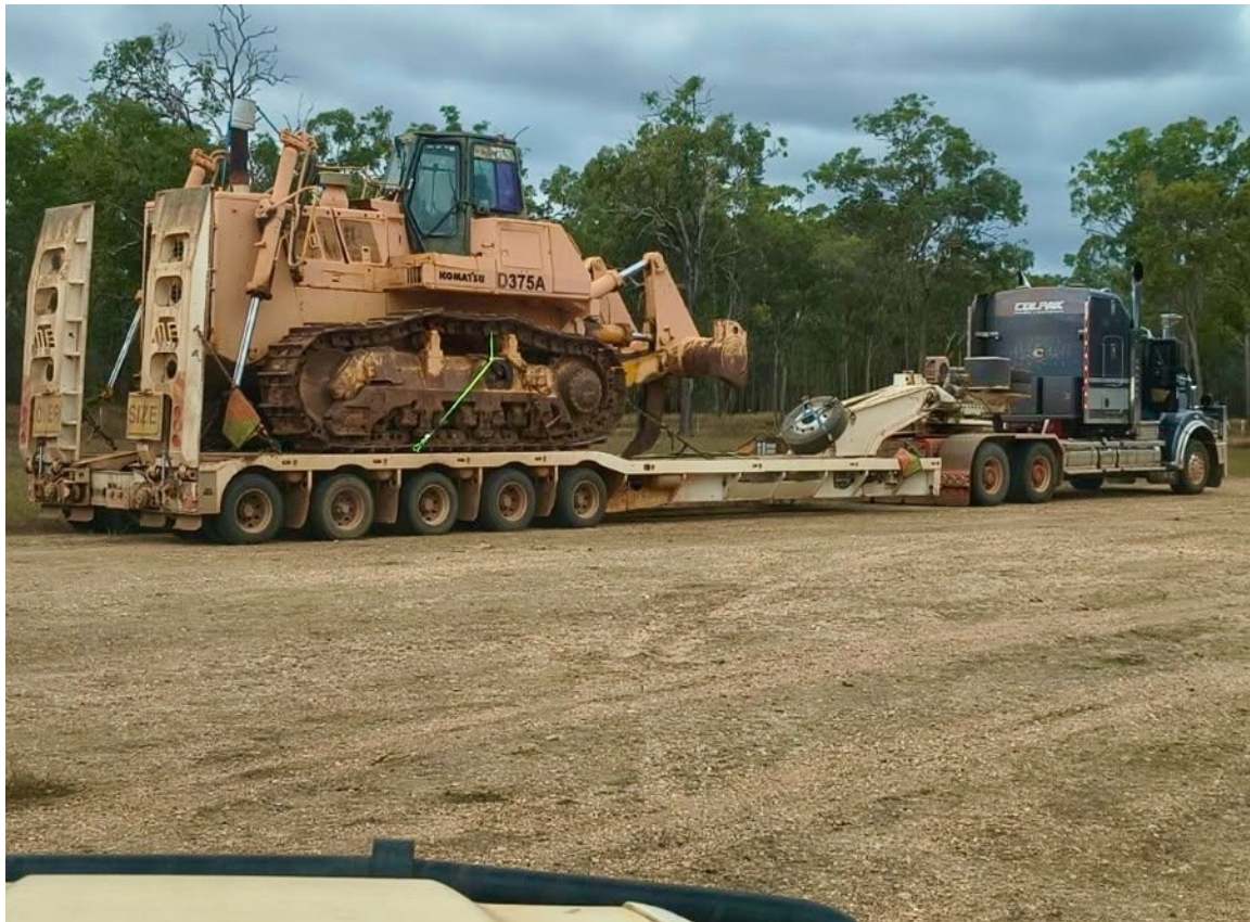
The first of GDM Challenger's open cut mining fleet mobilises, for final assembly on site.
